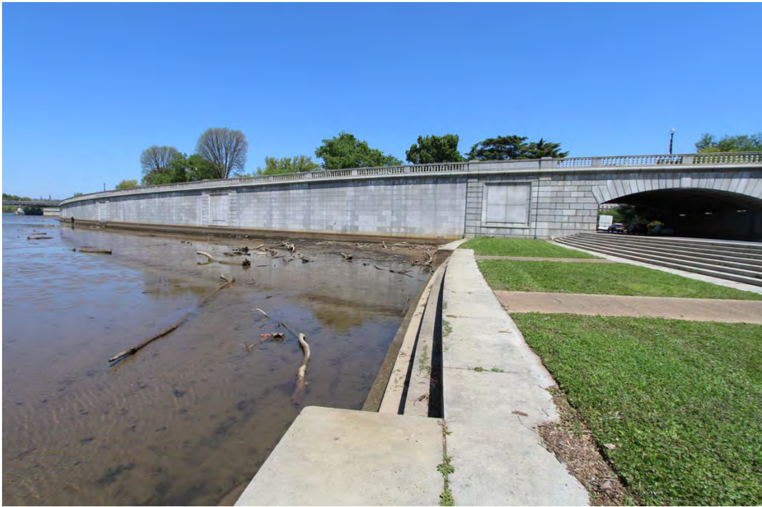
Fig. 90: View to the north of the historic Parkway Drive NW overpass and wall structure, containing the storage room (not visible). (Torkelson 2021)
