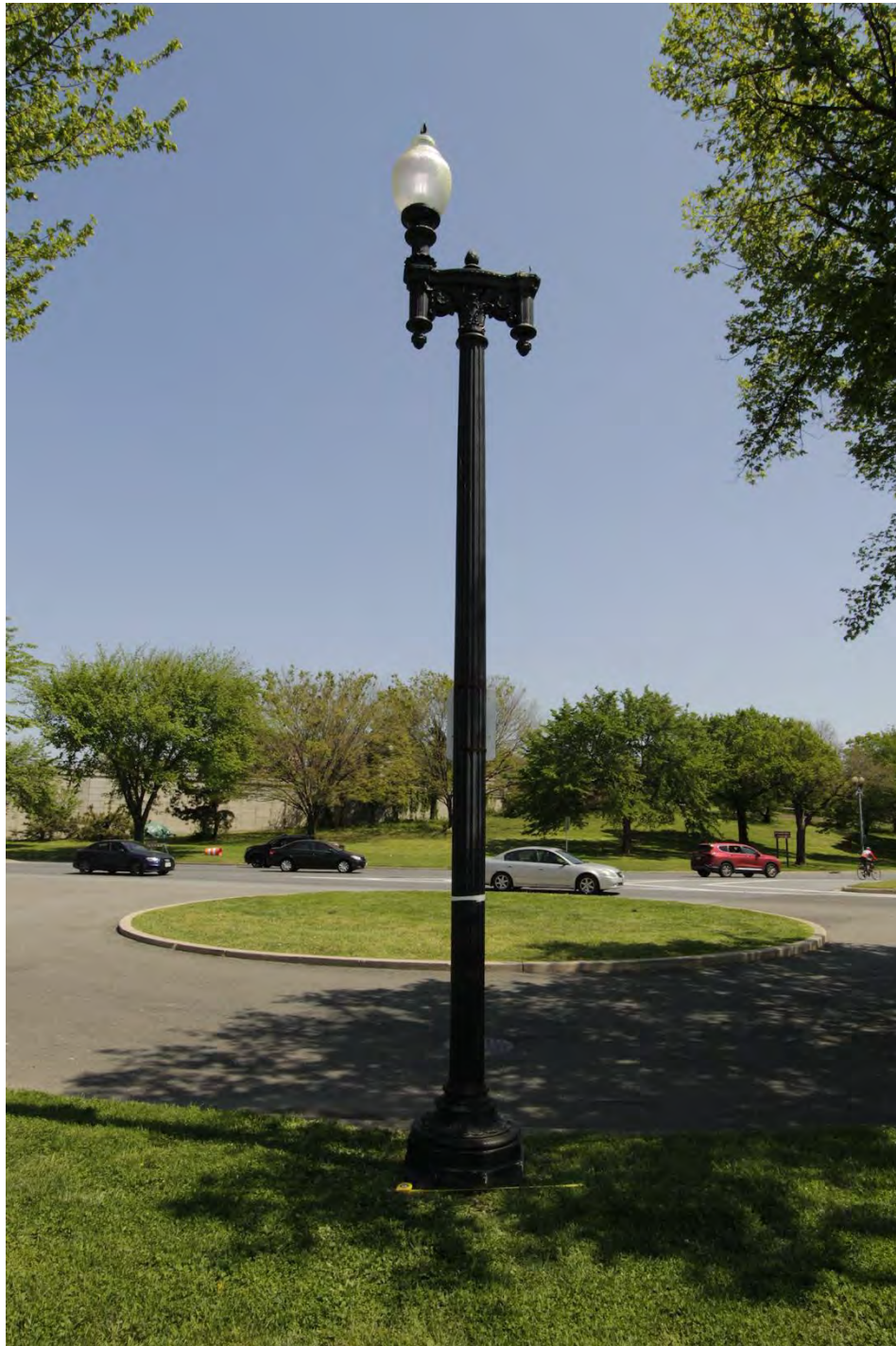
Fig. 109: Example of a Twin Twenty lamppost at the Belvedere. It retains its historic form, although the black paint color is non-historic (historically gray) and it is missing one of its luminaires. (Torkelson 2021)
