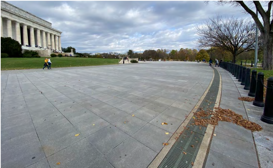
Fig. 72: View to the north showing the non-contributing (compatible) block paving and storm drains installed along the east side of Lincoln Memorial Circle at the new plaza. (Mason 2020)
