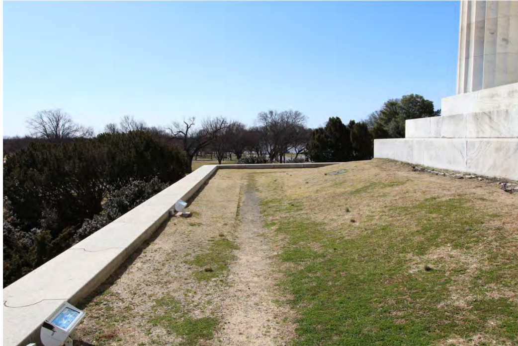
Fig. 73: View to the south showing the deteriorated historic gravel path along the edge of the raised terrace. (Torkelson 2021)
