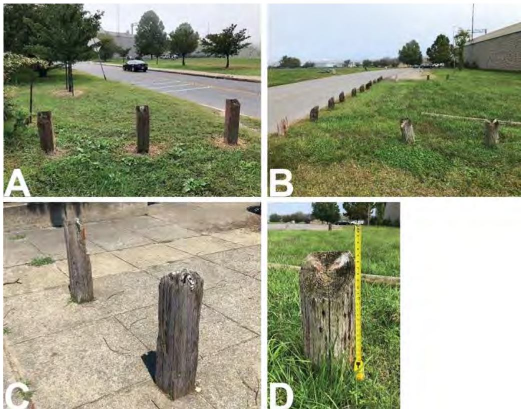
FIGURE 102a-d: Examples of wood bollards throughout the cultural landscape. A) View to the southeast of bollards along Good Hope Road SE in Section C; B) View to the northeast of bollards in parking lot C3 in Section C; C) Bicentennial-era bollards at the Section E playground; D) Detail of wood bollard in parking lot C3. (Photos by CLI author, 2019-2020)
