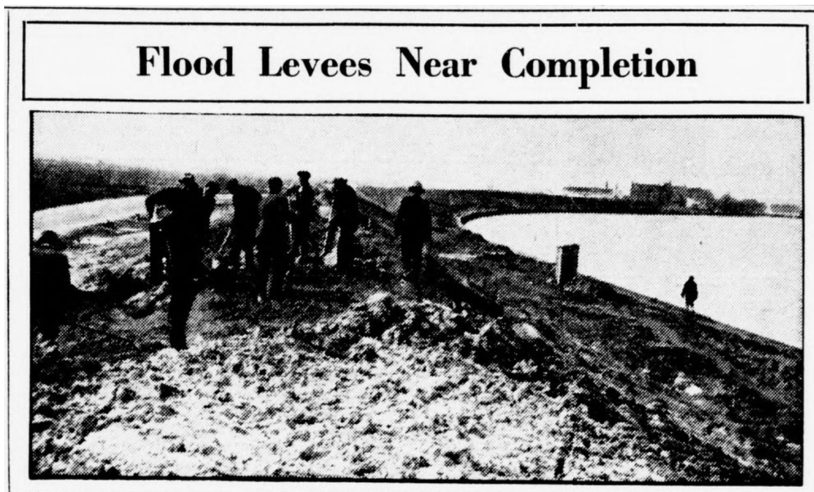
FIGURE 41: CWA (and later, WPA) workers were employed to level and improve land along the Anacostia River in Section C. In 1927, WPA workers constructed earthen flood levees beginning at Giesboro Point (south of Section C) and surrounding the tree nurseries in Section C. ( Evening Star , March 22, 1937: B1)
