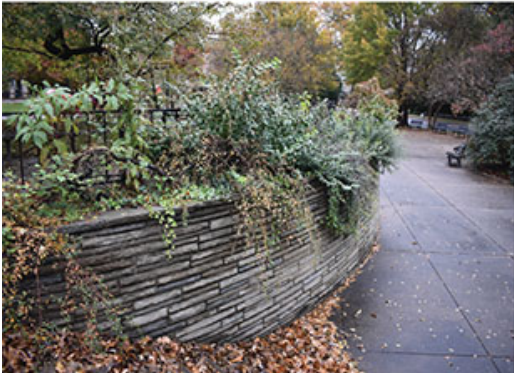
Existing vegetation conditions on the southwest terrace, including the little leaf linden tree (top) and the planting bed along the top of the radial retaining wall (bottom). (Photographs by the CLI author: top, March 2019; bottom: November 2018).
