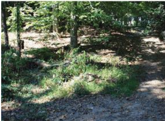
Views of the CCC-era amphitheater, including the concrete stage (top) and the deteriorated hillside seating (bottom), which retains traces of the rustic log seating that the Civilian Conservation Corps constructed between 1935 and 1937. (M. Lester 2015)
