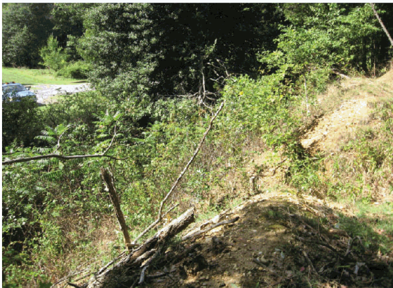
View of the earthworks from the parking area (top) & parapet wall (bottom). Erosion has more of an impact on this side of the fort due to tree removal. (CLP 2012)
