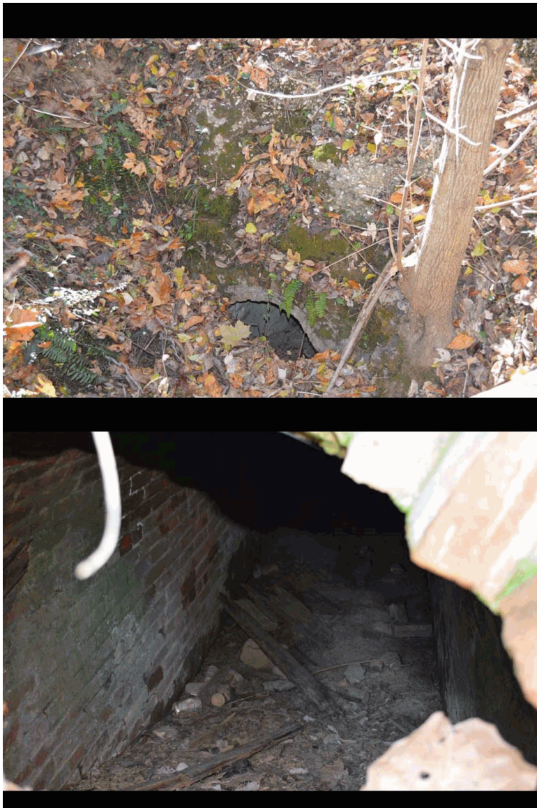
Fig 28 Upper: Culvert in the waterface of fort parapet, rediscovered during fieldwork for this CLI. Lower: Interior view of culvert (2014 CLP/NCR).
