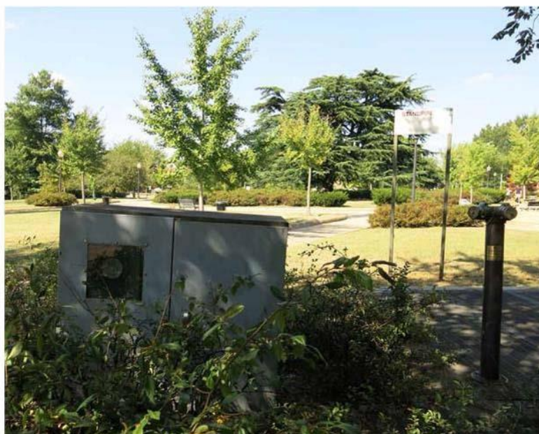
Figure 20: Metro signage (top) and stand pipe, meter and grate (bottom), installed within Grant Circle, Reservation 312.
