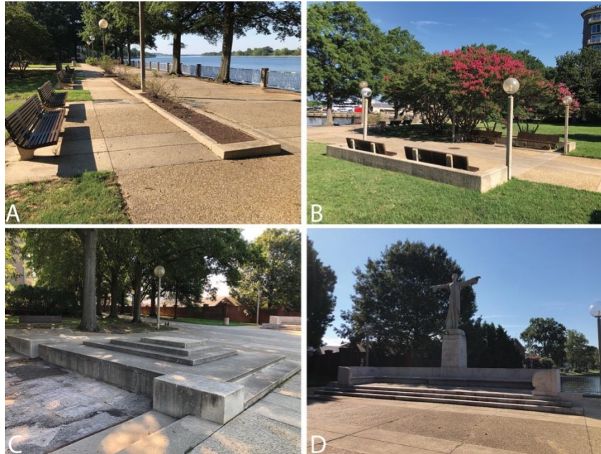
FIGURE 57a-d: Examples of historic structures that were installed during the primary period of significance (1967-1968): (A) planting bed structures along the NW/SE walkways; (B) low knee walls flanking the seating areas along the O Street SW walkways; (C) concrete stairs, walls, and steps in the south play area; (D) the Titanic Memorial sculpture located at the southern end of the cultural landscape. (Photos by CLI author, 2020).
